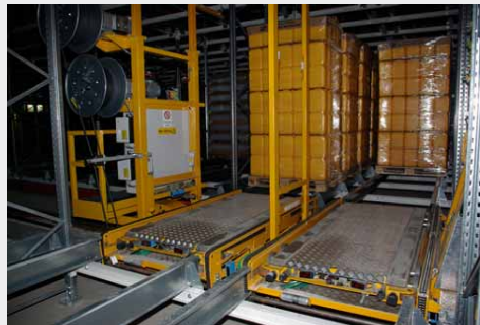
1 stacker crane with 2 channel vehicles.
